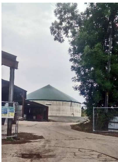
Figure 59 - Anaerobic Digester Wappingthorn Farm
